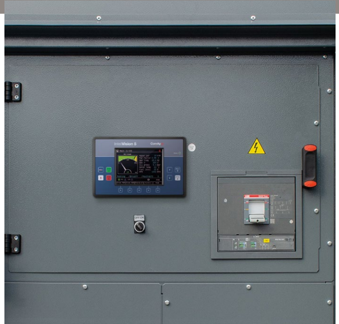
> Synchronization panel with ComAp IG1000 control unit
